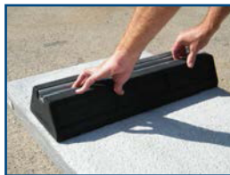
2. Place both feet on the light weight slab to match the pitch of ASHP feet.
